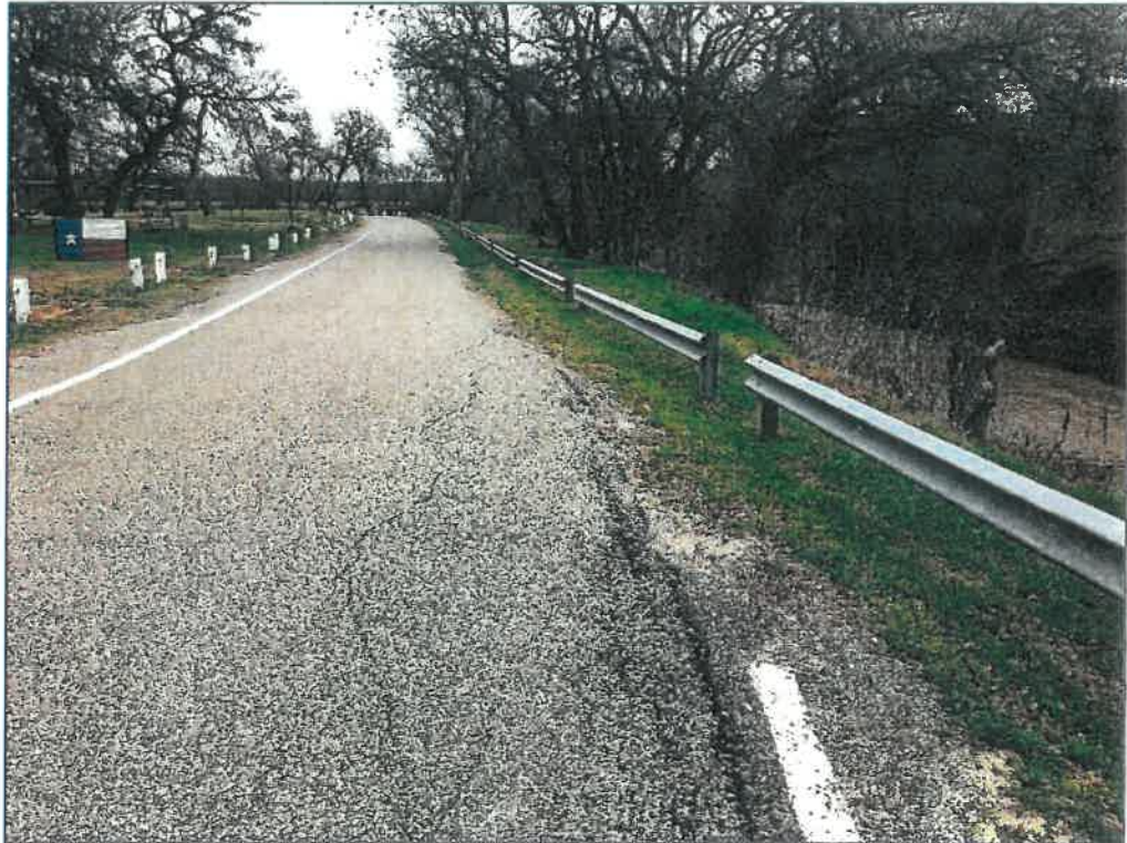
Figure 18: Slope failure damage to loop road pavement and subgrade
