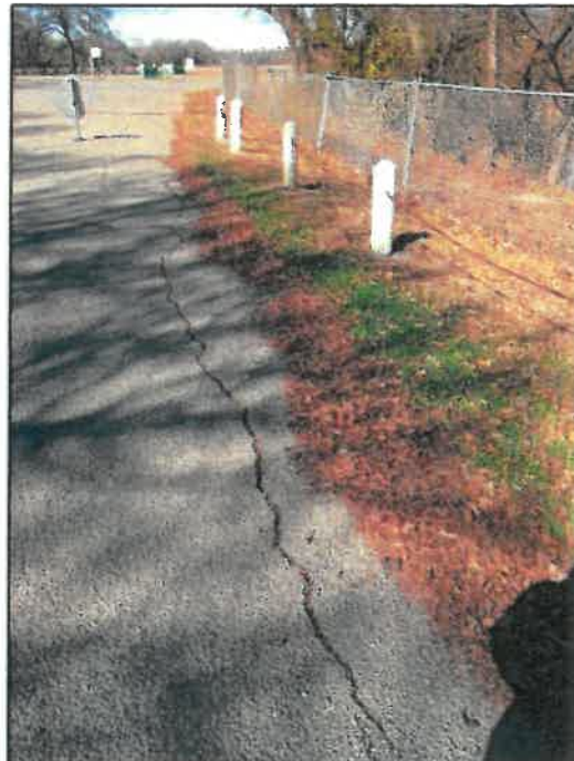
Figure 8: Pavement crack in loop road, looking downstream
