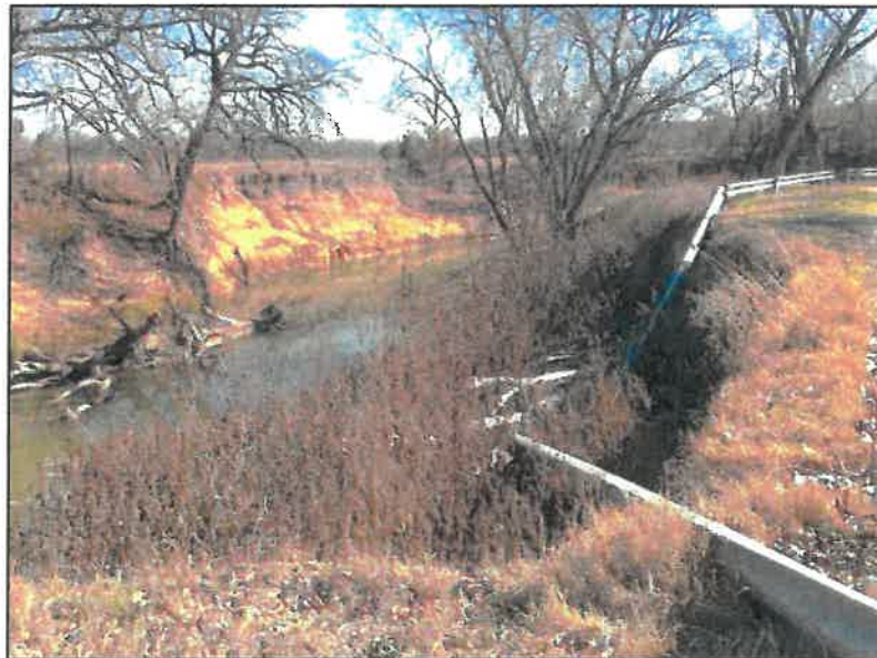
Figure 6: Slope failure and traffic barrier damage at end of park loop, looking upstream
