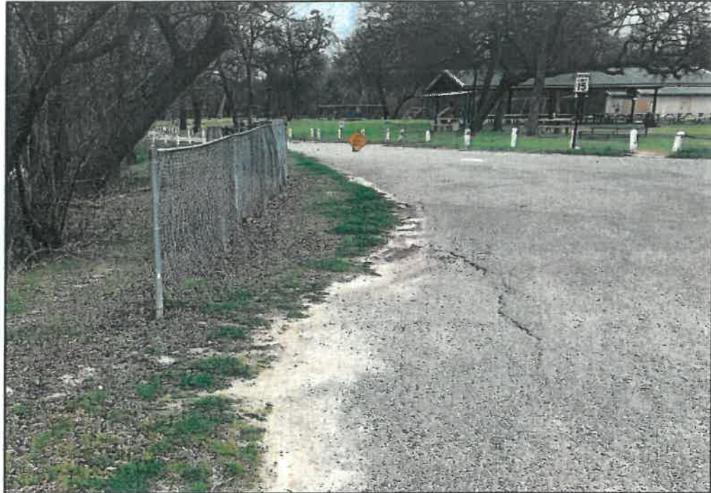
Figure 21: Pavement crack with vertical displacement near entrance to Faunt Le Roy Park
