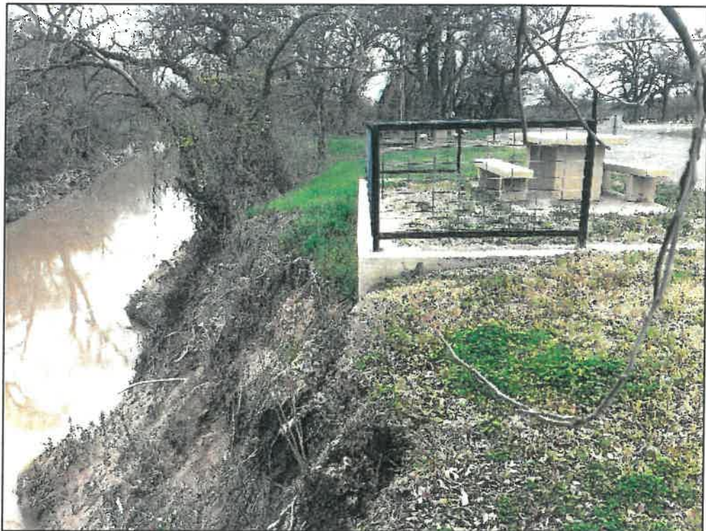
Figure 17: Slope failure damage to Leon River bank beneath Camp Site #6 picnic area
