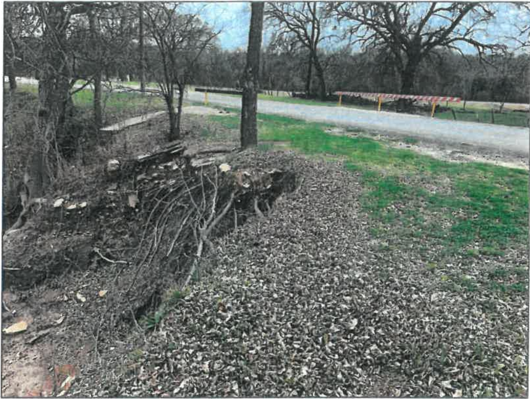
Figure 22: Surface water runoff scour of river bank, 7 th Street culvert crossing near park entrance
