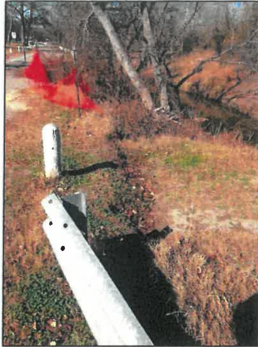
Figure 7: Slope failure and pavement damage, looking downstream
