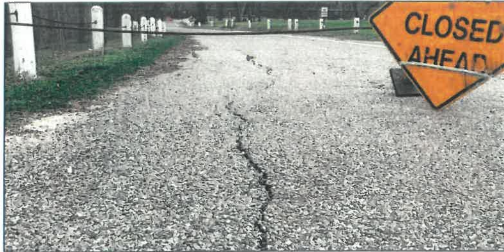
Figure 20: Wide crack in loop road pavement at barricade upstream of park entrance
