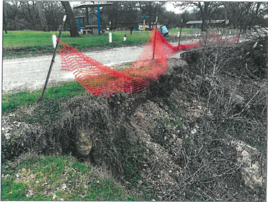
Figure 19: Slope failure damage to loop road pavement and subgrade
